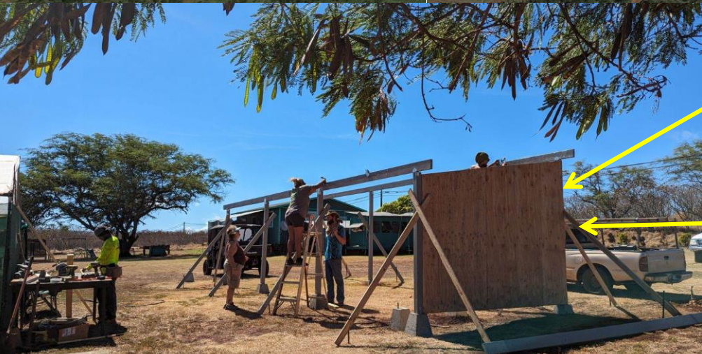
Off-Grid Canopy Ground Mount
