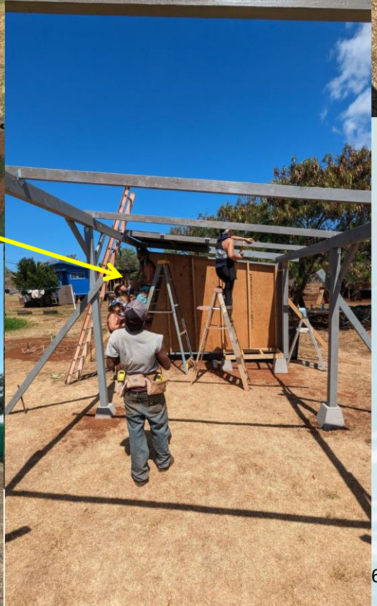
Off-Grid Canopy Ground Mount
