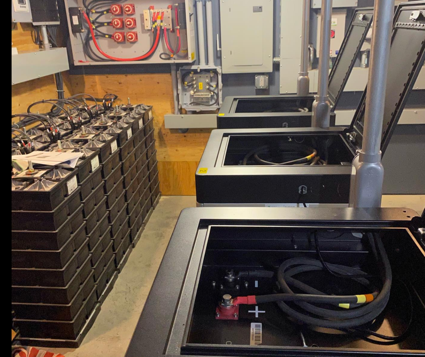
First three eVaults sharing the load with the Aquions
