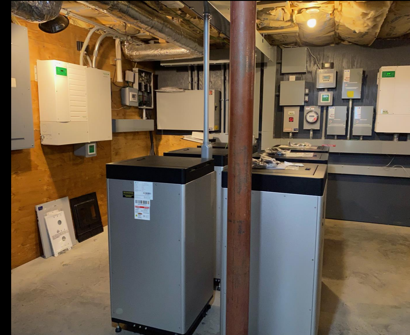
Finally 6 Fortress eVault Max 18.5kWh batteries (110 kWh) Aquions gone.
